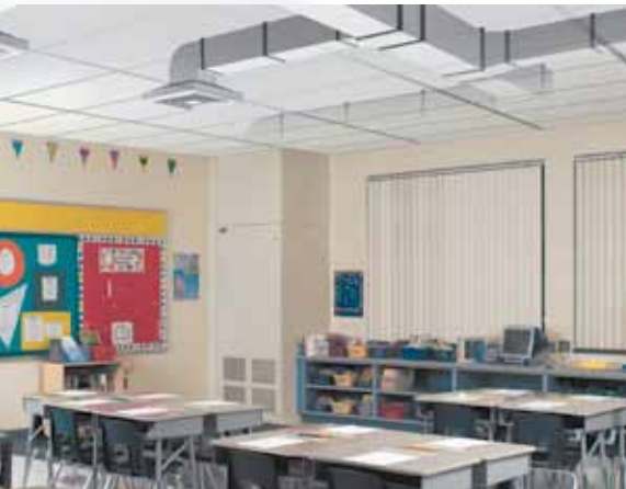
Supply air is ventilated throughout the classroom via a ducted ceiling system in this example.
